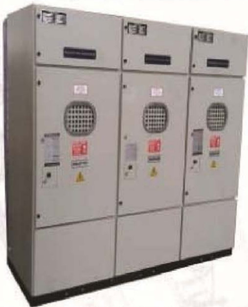
RING MAIN UNIT WITH VCB AS T off AND TWO AIR INSULATED LOAD BREAK SWITCHES AS INCOMERS.
