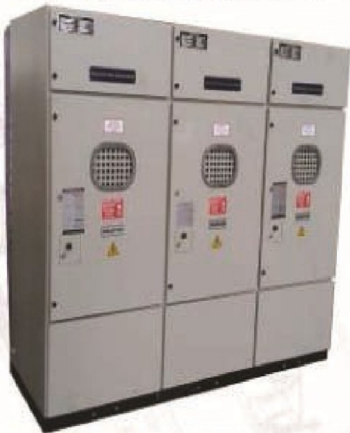
RING MAIN UNIT WITH VCB AS T off AND TWO AIR INSULATED LOAD BREAK SWITCHES AS INCOMERS.
